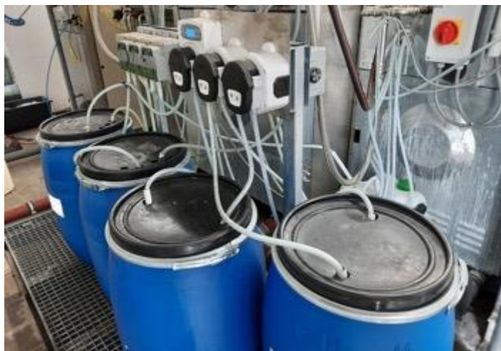
Figure 13: Example of a closed automated dosing system for garment finishing washing machines
