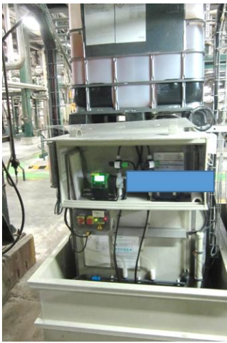
Picture: IBC with liquid enzyme on their secondary containment; example of mother- daughter decanting system
